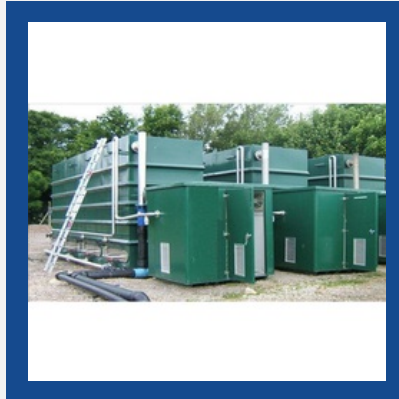
Effluent Treatment Plant
