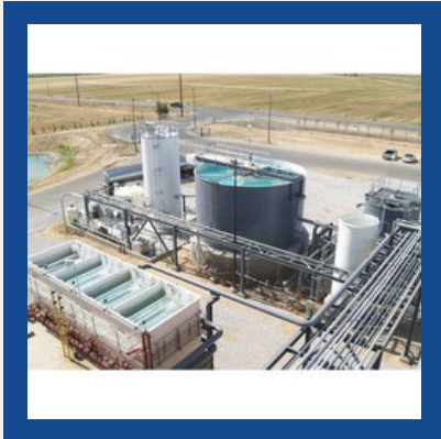
Zero Liquid Discharge Plant
