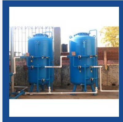
Water Softening Plant
