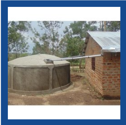
Rain Water Harvesting System
